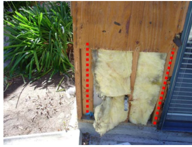
Figure 2: Missing hold-downs (red dotted lines indicate intended locations)
