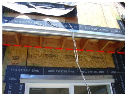
Figure 5: The red dashes show where shear transfer clips should have been installed
